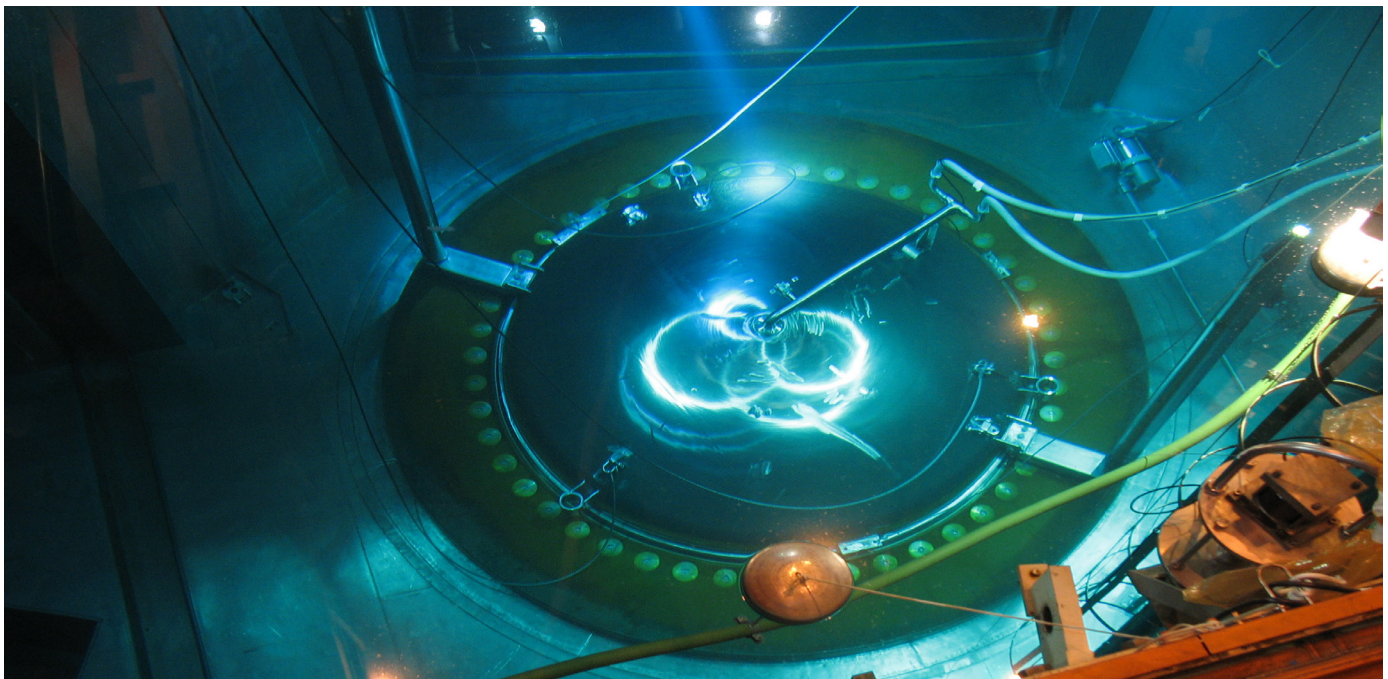
Figure 1: A Temporary Reactor Head installed during a maintenance outage
