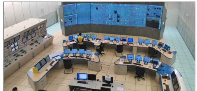
Full-Scope Nuclear Power Plant Control Room Simulator
