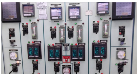
HMI units with their touchscreen counterparts.
