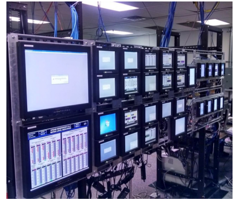
Touch-screen panels on the new control board mimic the former analog displays.
