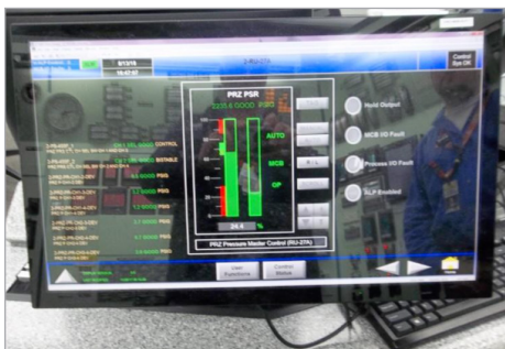
Example of HMI workstation.
