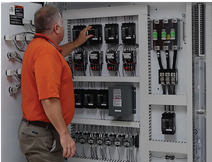
HVAC Electrical Control Panel
