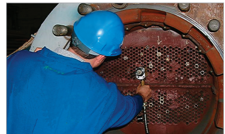
Heat Exchanger Field Service
