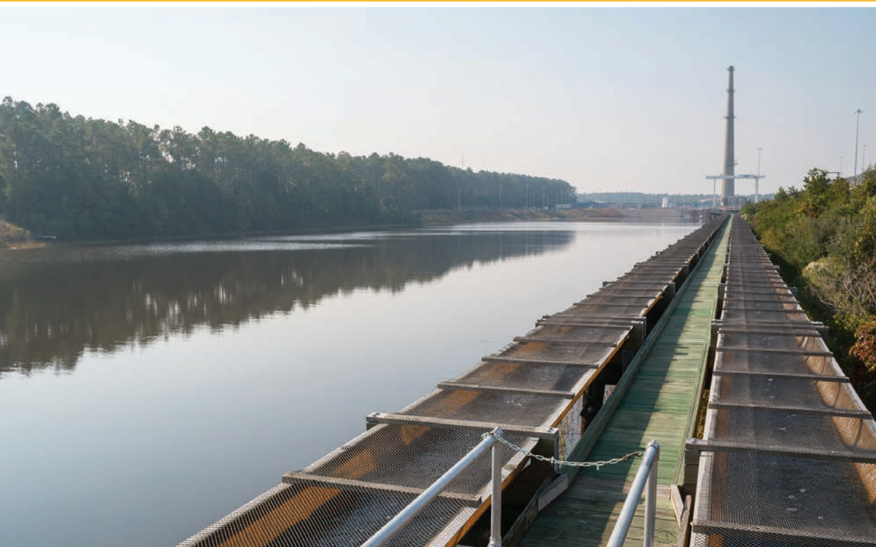
The intake canal for the Brunswick Nuclear Plant features the “Slide for Life” which is used to minimize impacts on local aquatic life.
