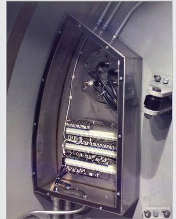
Airlock EPA with Junction Box
