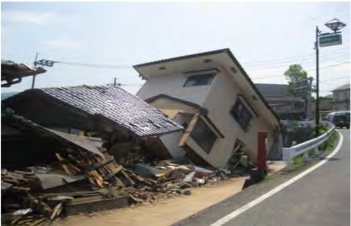
Soil slumping or spreading caused some collapses, as with this home that tilted toward the nearby stream bed.
