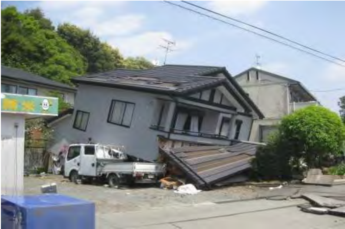
Collapse of homes was often attributable to soft first stories containing garages where large door openings provided no restraint against lateral loads.
