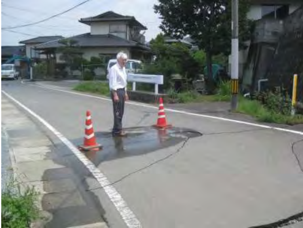
Rupture of underground water mains delays restoration in soft soil areas subject to severe shaking. The photo shows water seeping from a break on the fault trace on the north side of the Mashiki Valley.
