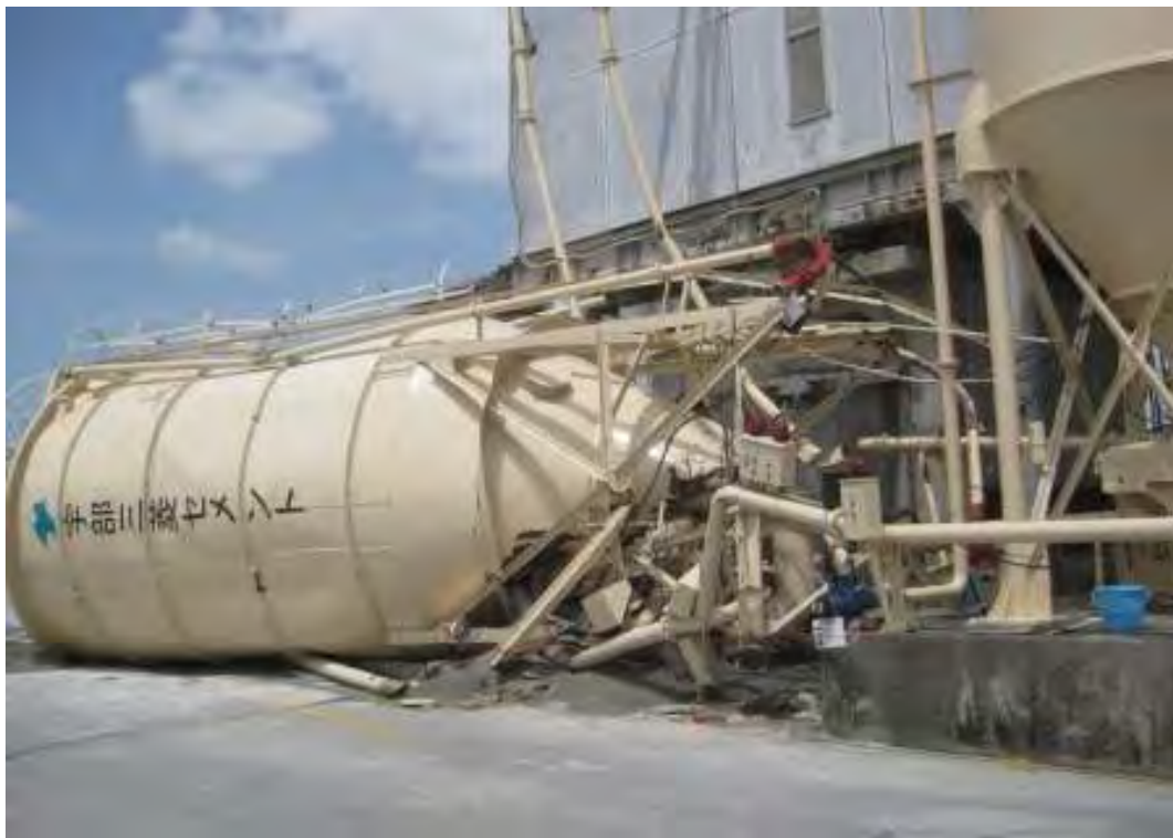
The two larger silos collapsed at a cement distribution plant southeast of Kumamoto. Overturning appeared to be caused by failure at flanged connections in the framing due in part to corroded bolts. The three smaller silos that remained intact and upright were reported as newer installations.
