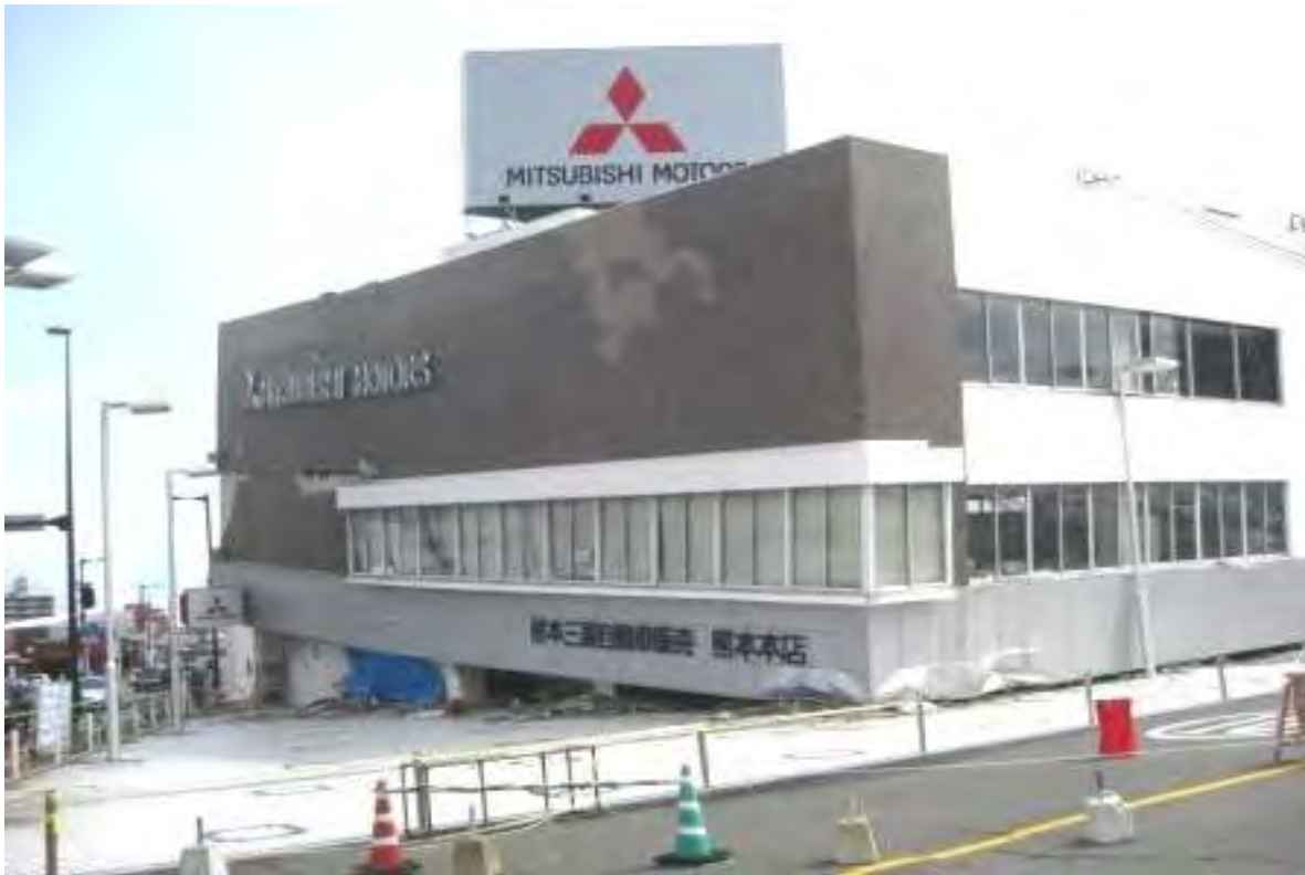
One of the few notable exceptions of serious building damage was the soft storey collapse of the Mitsubishi dealership show room in south central Kumamoto. Lack of adequate ties around vertical rebar in the concrete columns appeared to be the root cause. The photo was taken just before the team was asked to leave by the Mitsubishi sales manager.
