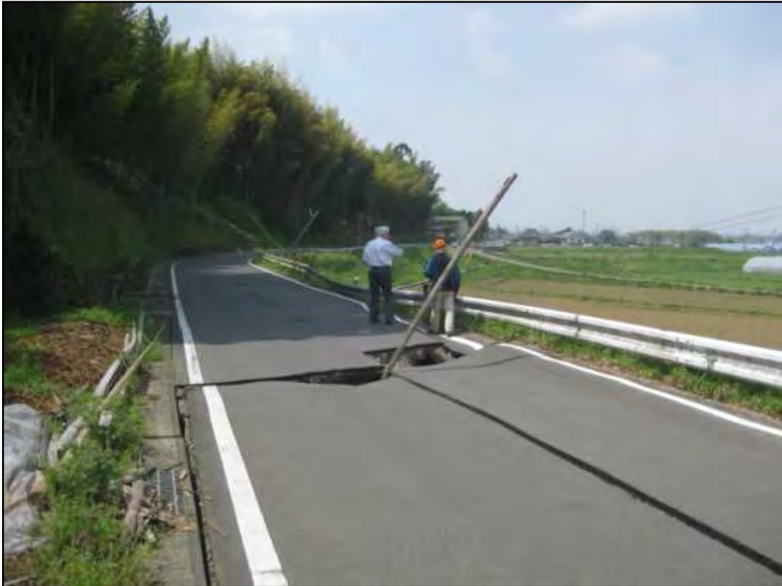
The fault rupturing the surface on a road in Mashiki Town
