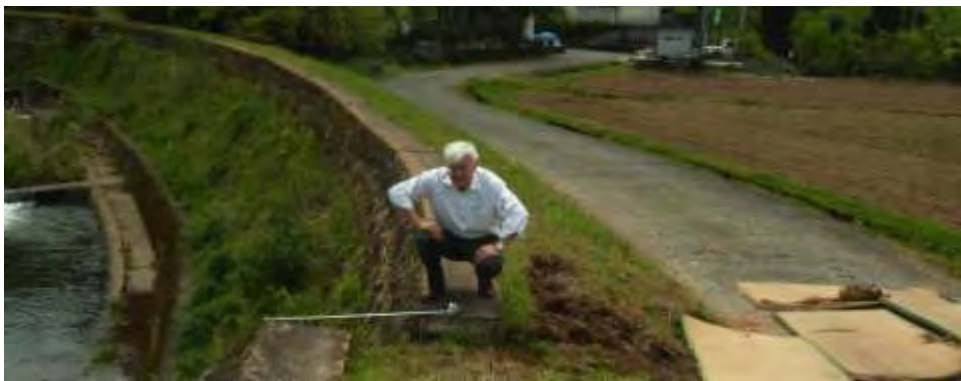
Faulting, along the Futagawa fault through a hilly residential area of Mashiki. At this location the fault has offset a retaining wall about 4 feet (1.2m). Houses founded right on top of the fault were typically completely destroyed. Nearby wood frame houses, not directly on the fault, had various degrees of structural damage – from light to extreme, including many collapses.
