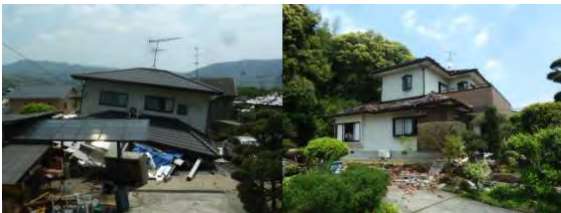
Other severely damaged houses in Mashiki. Most of the damage that occurred was due to too many windows and not enough strength in the lower floor walls. That additional strength can be easily provided with the bracing provided by a few more well-nailed plywood sheets.
