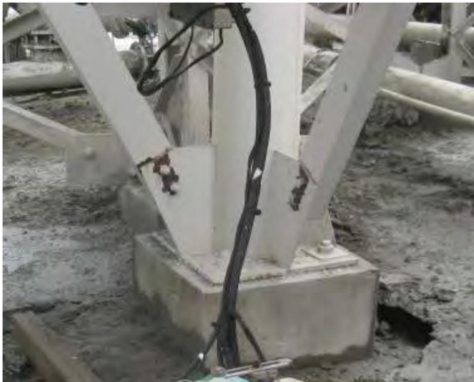
A cement silo at a distribution plant southwest of Kumamoto was being re-leveled by crane lift six days after the earthquake (upper photo). Drop of one corner of the silo foundation pedestal due to soil settlement (lower photo) lifted the opposite corner.
