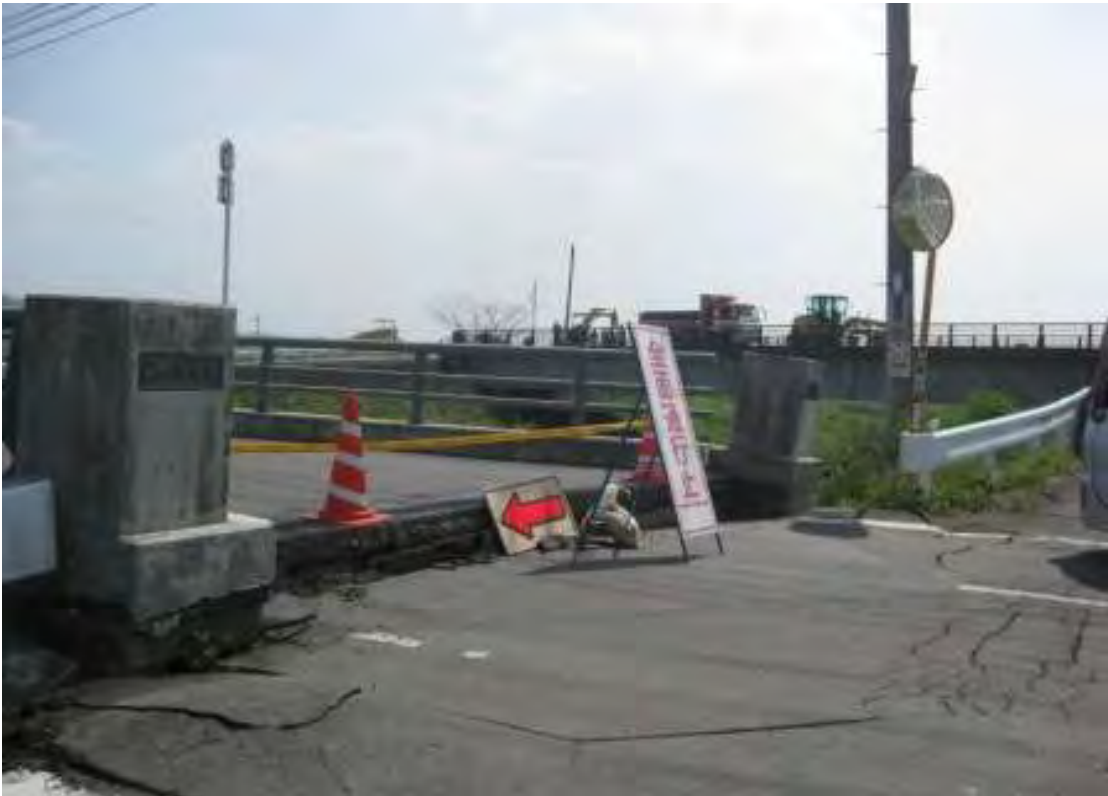
Traffic arteries were closed following the earthquakes due to bridge and overpass damage including failure in columns (upper photo) and slumping where bridges meet abutments (lower photo). Closures divert traffic to alternative routes creating major delays that affect the population far beyond the area of earthquake damage.
