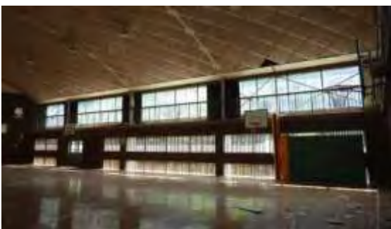
Interior of the virtually undamaged gym. A few lightweight ceiling tiles fell because of inadequate attachment to the structural roof (and ceiling). The debris can be seen in the lower right corner; all the windows are intact.
