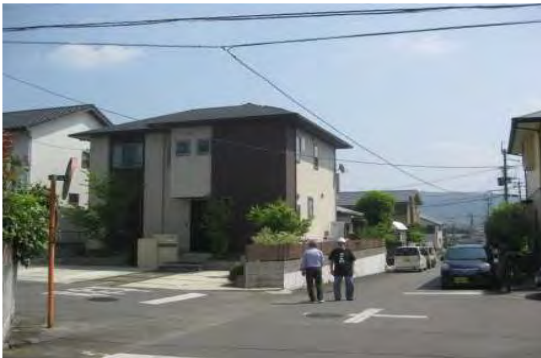
Serious damage was sporadic in the newer homes of the residential area on the hilltop near the Mashiki strong motion instrument. Close inspection however revealed that most homes required some level of repair. Damage became more extreme proceeding down the hill into the older district atop softer soil.
