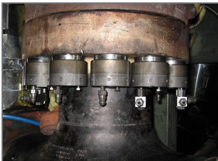
Main Steam Relief Valve – BWR Plant
